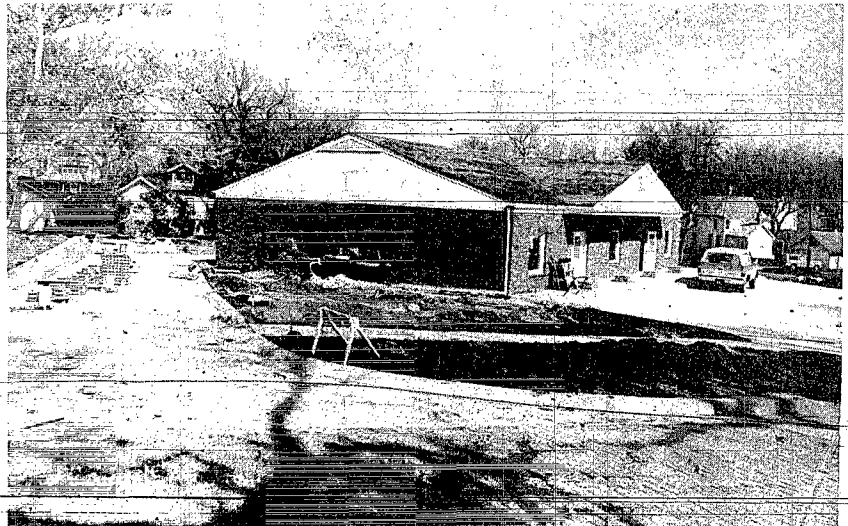
CONCRETE DRIVES , with curving lines, are the recent visible progress at the new office of Columbus Federal Savings and Loan Association. Other construction continues inside and out.
